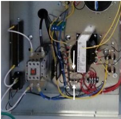
Fuses FS10 and F11 are located on the panel near the control transformer
