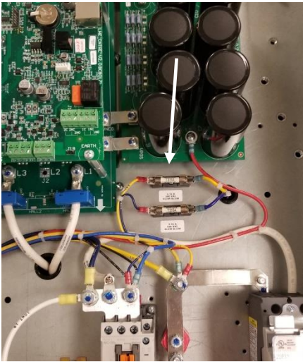
Fuses FS10 and F11 are located on the panel near the circuit breaker.
