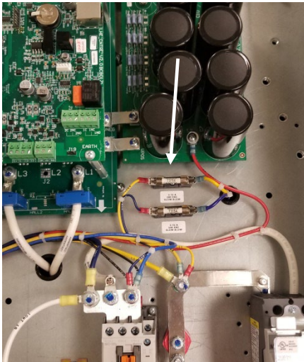
Fuses FS10 and F11 are located on the panel near the circuit breaker.
